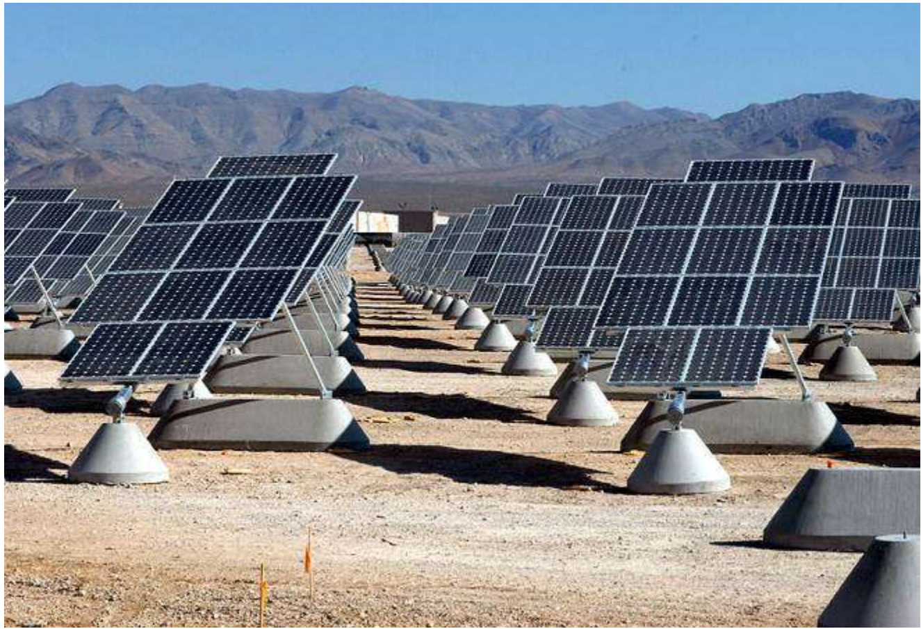
Figure 2: Tracking PV array
