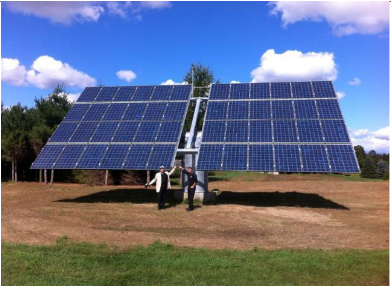
Figure 3-2: Tracking PV array (sourced http://solarblog.ca )
