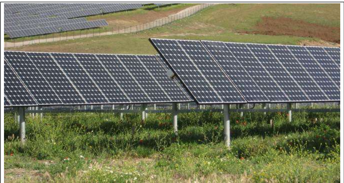
Figure 1: Fixed tilt PV array
