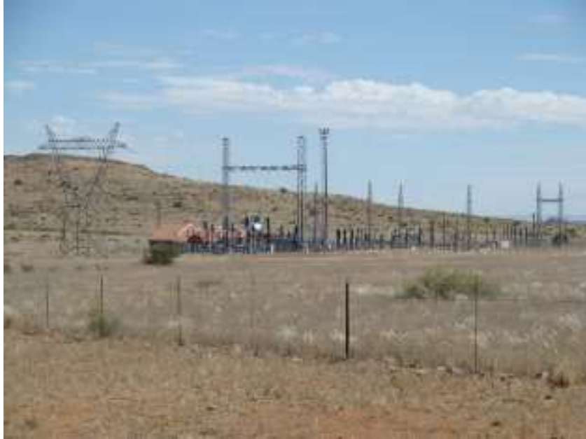
Figure 4: View of ESKOM's Paulputs Substation from the assessment area.
